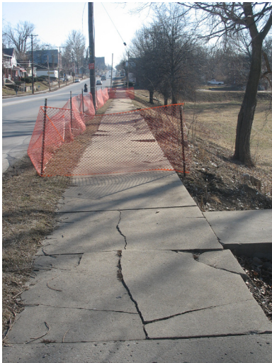
Dangerous sidewalk conditions on Prospect near 19th Street. Neglected maintenance of infrastructure is a problem throughout the neighborhood.
