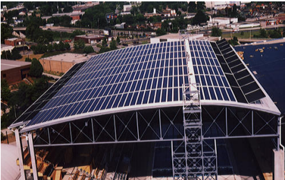
Rooftop Solar Energy
